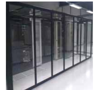
Centralized Cooling Adaptation
